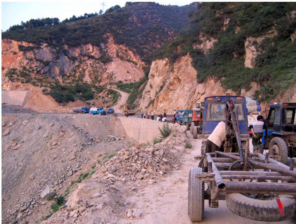
Traffic Jam at the Shitou Dam
